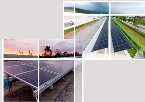
Panasonic Kulim, Malaysia 1 MWp ground mount solar PV
